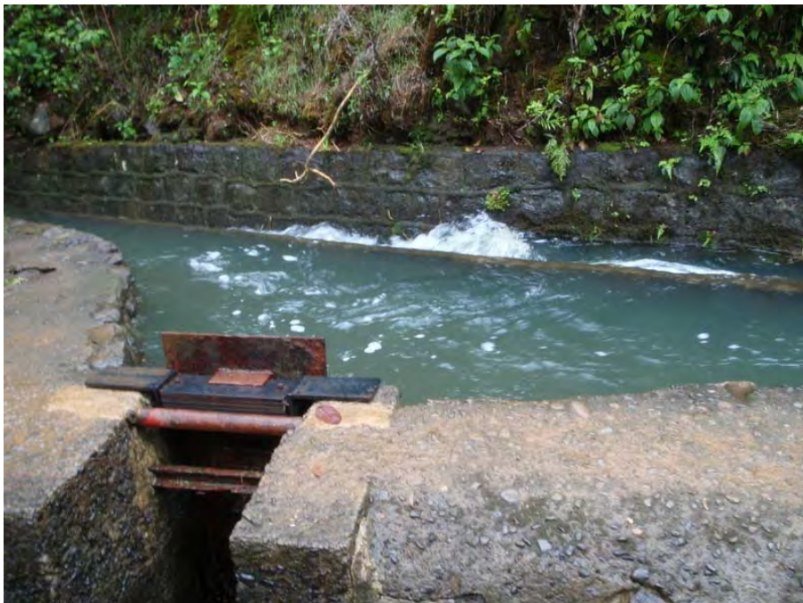
Control gate water flowing into stream (gh002d-022p-041012)
