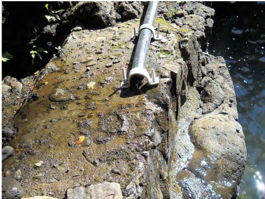
Not effective in providing connectivity at low flow
