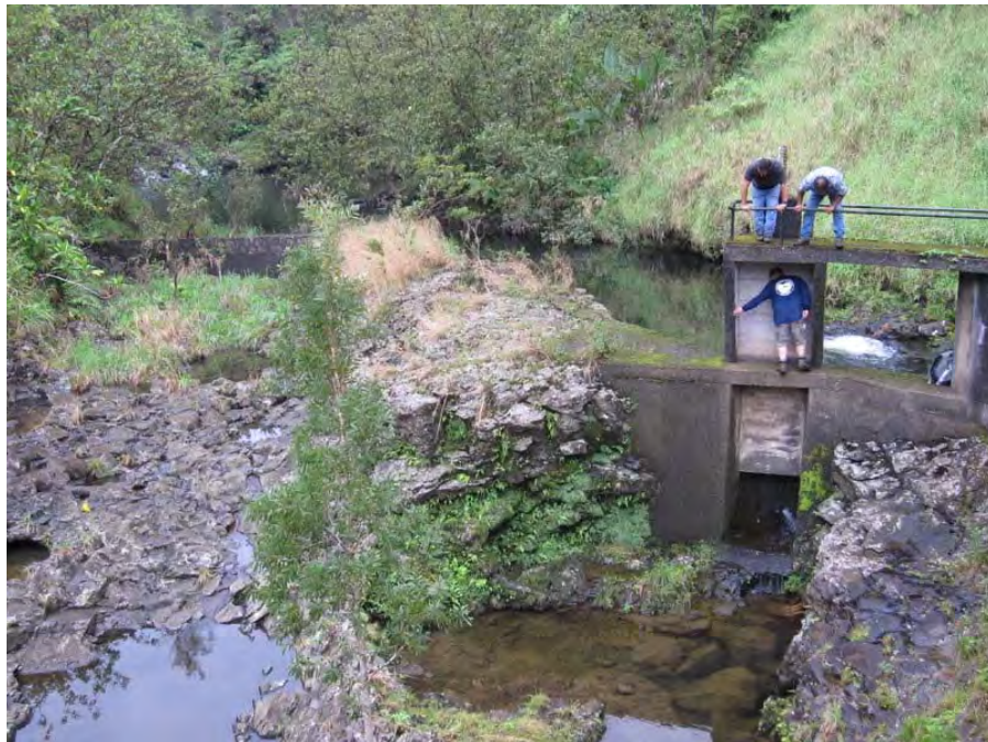
Upstream view from bridge of the diversion (right) and dam wall (left)
